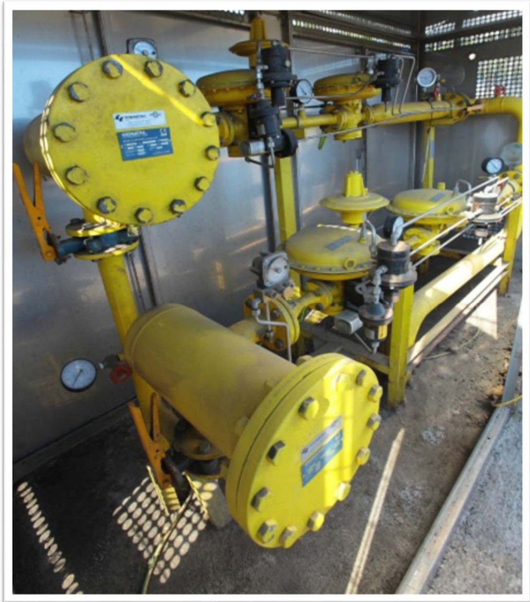
Giarre – Decompression Station
